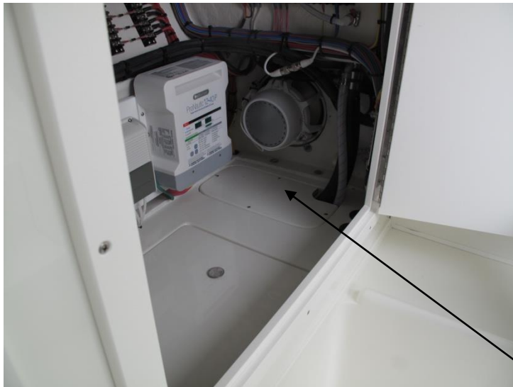
Port Tank Sending Unit
